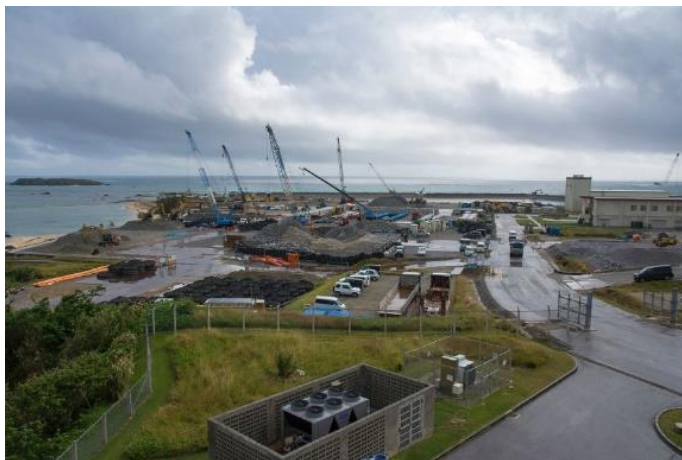
Construction equipment is seen near Oura Bay at Camp Schwab, Okinawa, Dec. 4, 2018.
