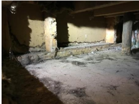
Mold damage is pictured in the house of senior airman Abigail Courtney at Tinker Air Force Base, Oklahoma, U.S. in this undated handout photo
